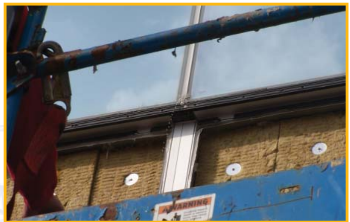
Trapped water escaping when a blocked weep is opened.
